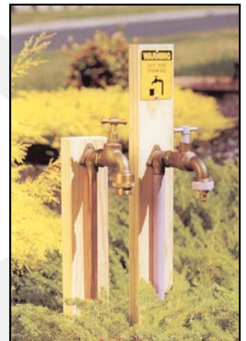
Dual supply system taps
